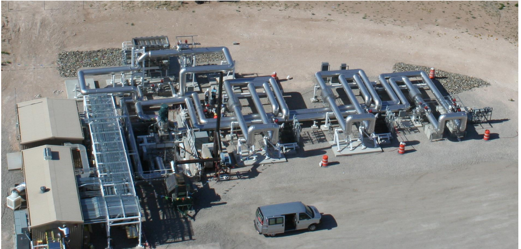
Sandia's Molten Salt Test Loop ( MSTL) MSTL is currently waiting for a restart of the loop
