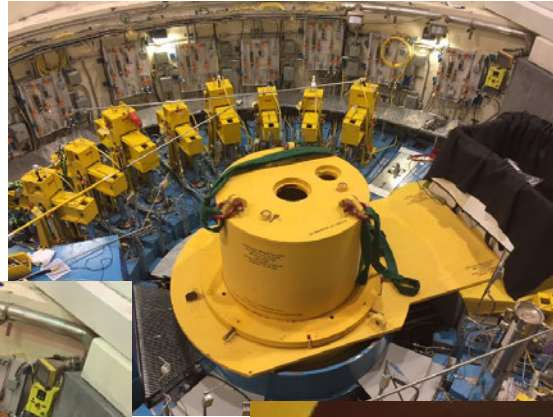
Shielded Cask in Position over Core Vessel
