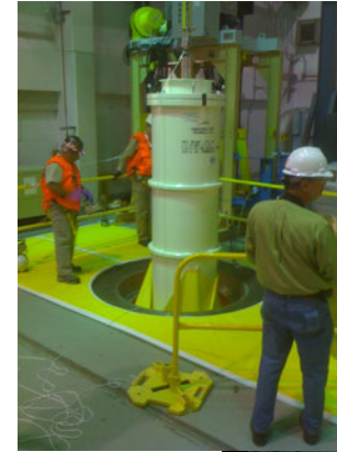
Loading a Liner into cell via Top Loading Port
