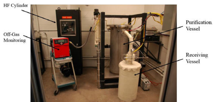
FLIBE WALK-IN FUME-HOOD WITH HF PURIFICATION
